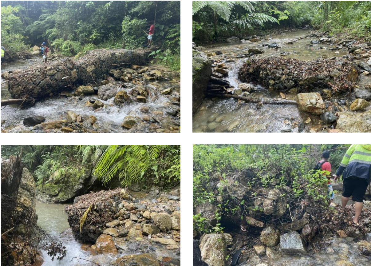
Figure 3. Images of the destroyed gabions in the Napaan River Watershed from an ocular inspection conducted last 07 June 2023. Engineering and Zoning Offices, LGU Malay
