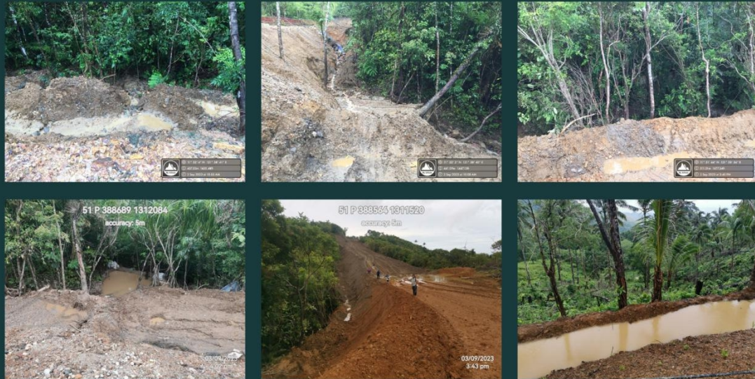
EARTH CANALS - POOR MITIGATION
